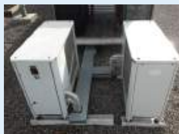
Back-up redundant systems
