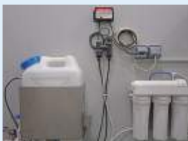
Water treatment systems
