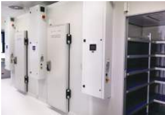
STABILITY ROOMS TURNKEY PROJECT BY ARALAB
