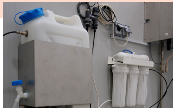
Water Treatment systems
